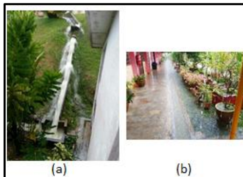
Figure 1 (a) Drainage at steep hill during heavy rainfall; (b) Drainage system with excess rainwater.
